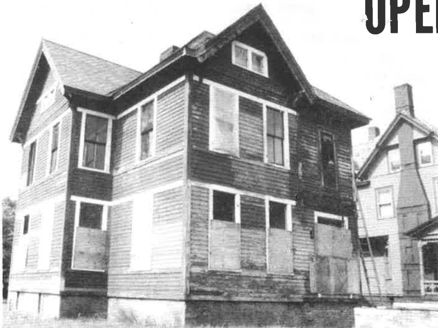
RESTORATION IN PROGRESS: the original porch was removed and has been rebuilt.
