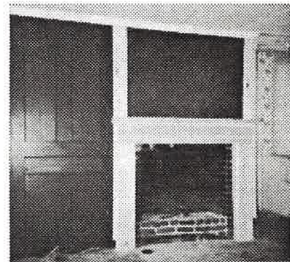
This 1840's firebox had been covered over in a 1950's renovation and was found while stripping off a 1970's Z-Brick wall.
